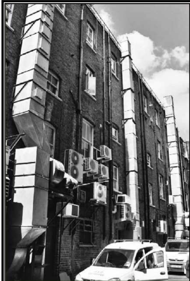
Figure 2.7: Ducting has a significant impact on the courts and alleys of Soho and Chinatown
